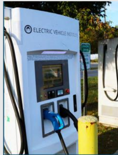
Figure 13: EV charging station (MDOT).
